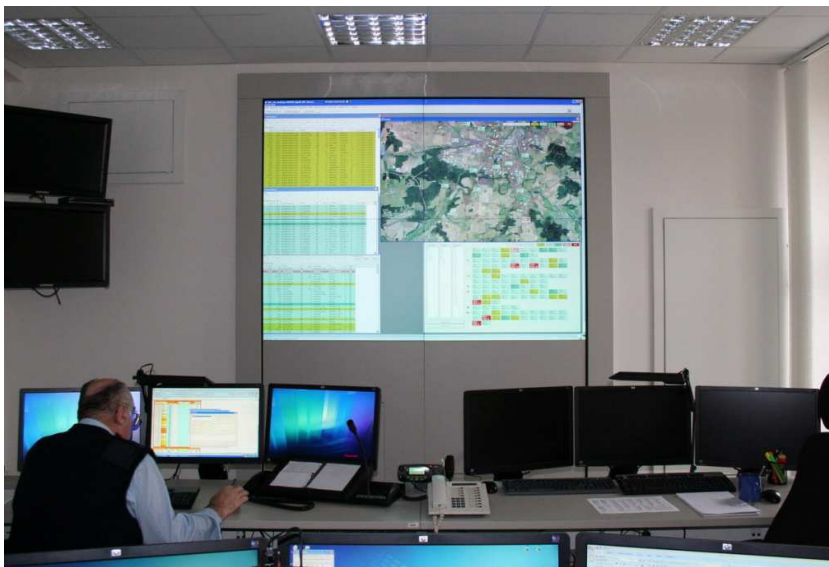
Pic. 2: The dispatcher center with central monitor
